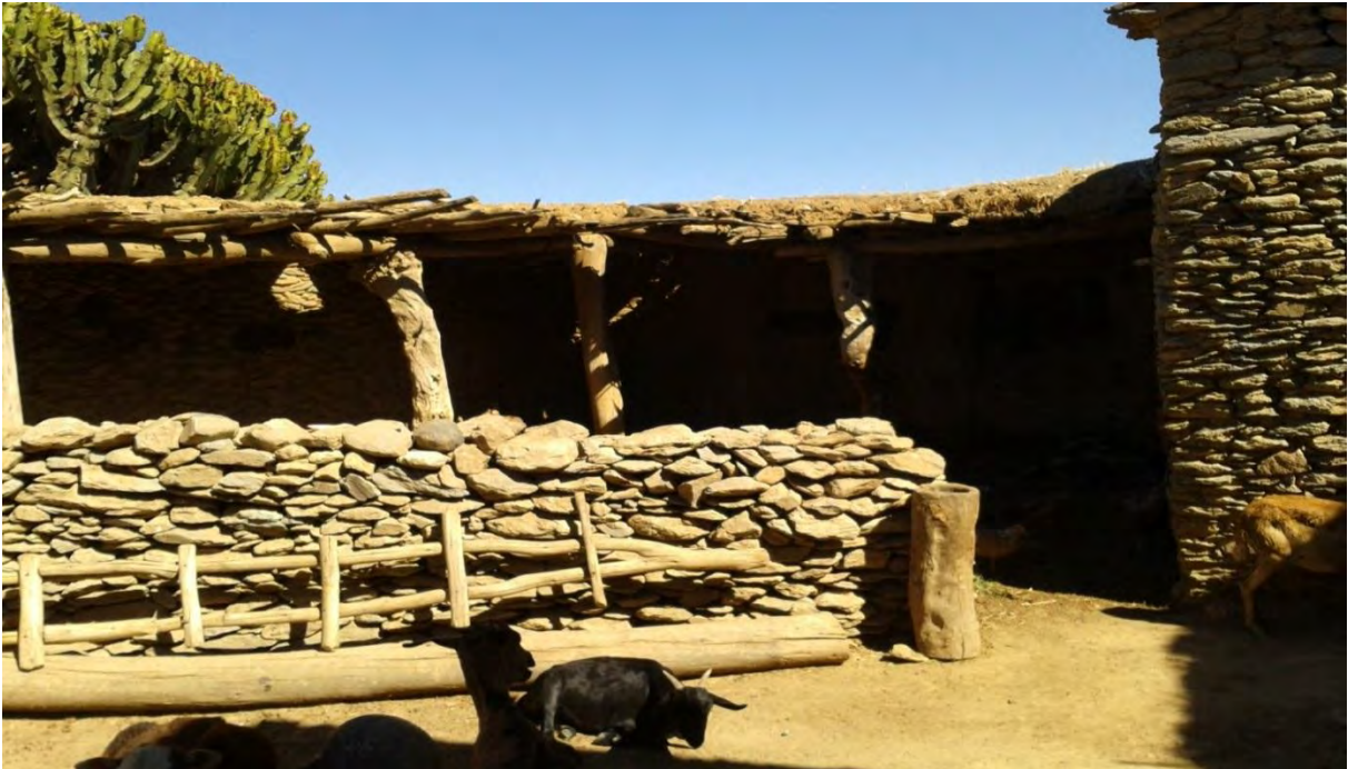
Figure 8.5: IFALE participant’s house in Tigray with a separate shelter for domestic animals
